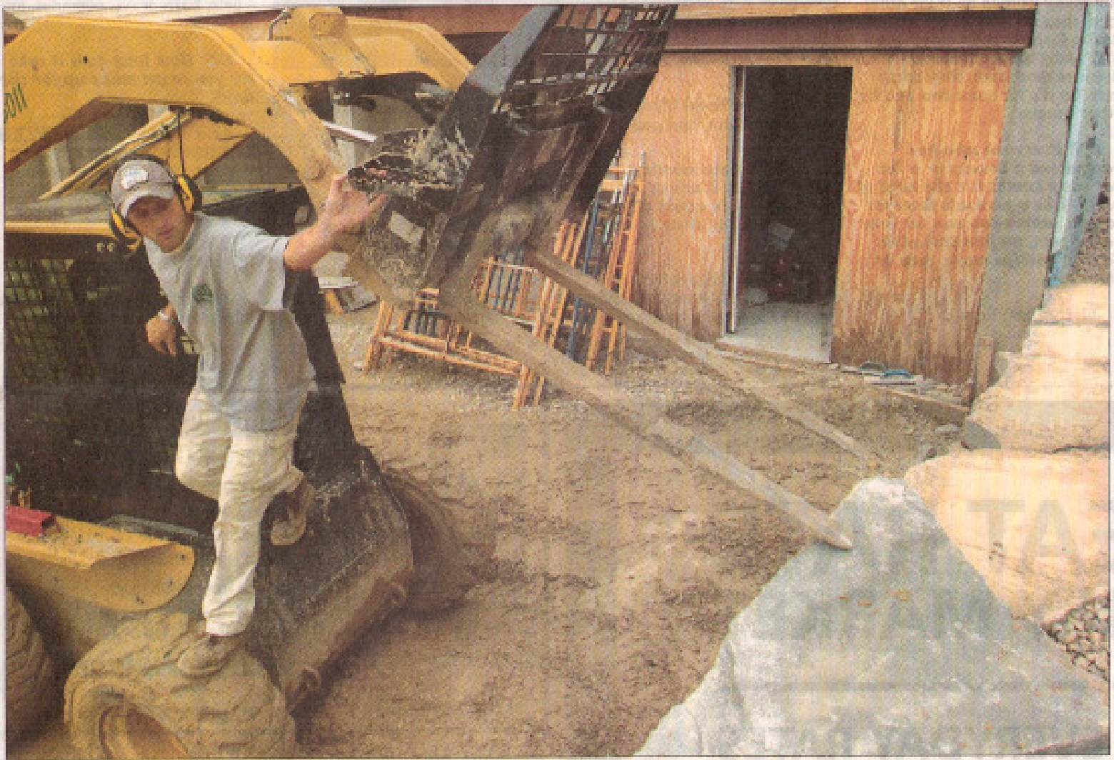
Margo Cohn Pactanac/Daily News Staff Forrest Peterson of Hartford works to put up a Lannon stone wall outside a new four-unit condominium building during the Habitat for Humanity home building blitz on Wednesday afternoon in West Bend. Peterson is with Extra Mile Landscaping. The construction on the building is expected to be completed in November.
